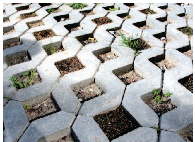
Fig. 8 One of the courtyards at Flagghusen, Western Harbour, Malmö, is to a large extent built with permeable concrete blocks. The permeability helps in reaching the required Green Space Factor, but most people would agree that the courtyard has low aesthetic value
